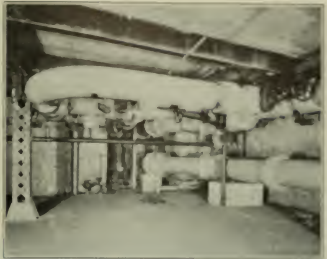
FIG. 16. DRY- AND EXHAUST-STEAM CONDENSER AT ENTRANCE TO TUNNEL
